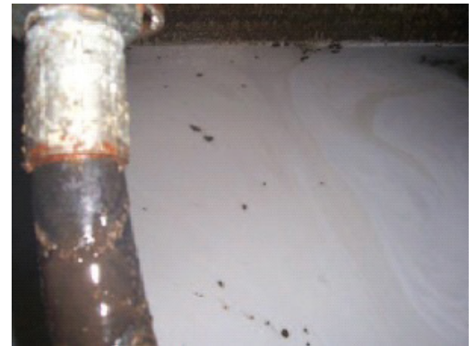
Before using QUINTOLUBRIC® in the longwall tank.
